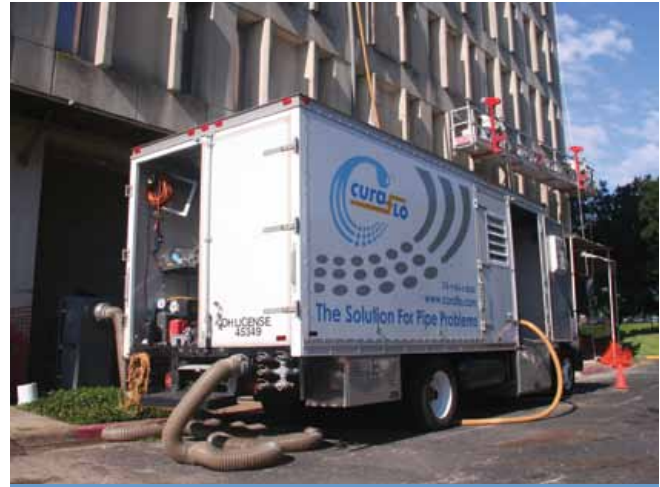
CuraFlo uses state-of-the-art equipment to complete lining projects as effectively and quietly as possible.
