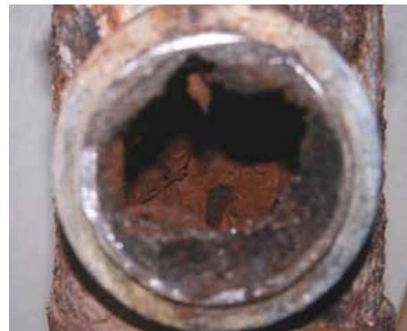
Tuberculation or build-up of scale inside a galvanized pipe reduces internal pipe diameter, consequently affecting water flow and water pressure
